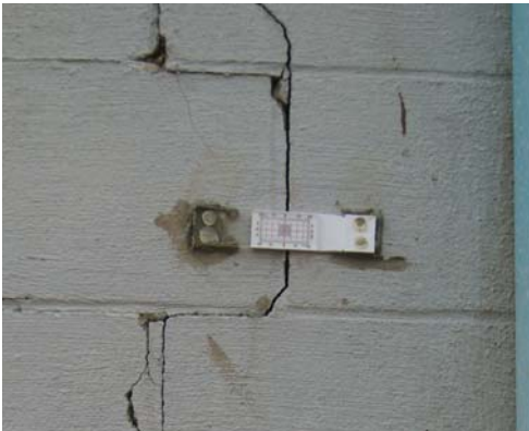
Monitoring existing wall crack
