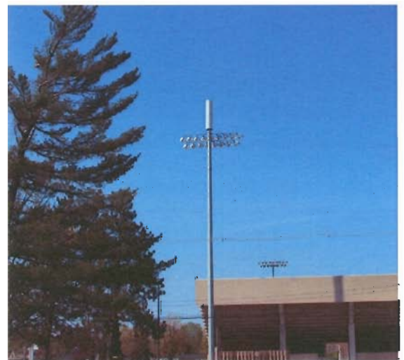
Antenna mounted on an athletic field light pole
