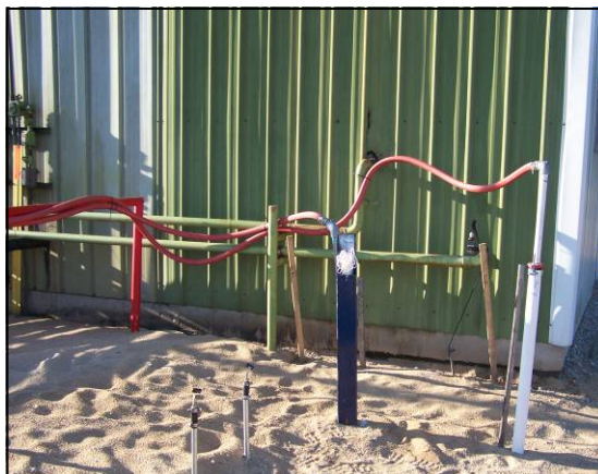
Photograph of monitor wells, biovent wells and monitor points.
